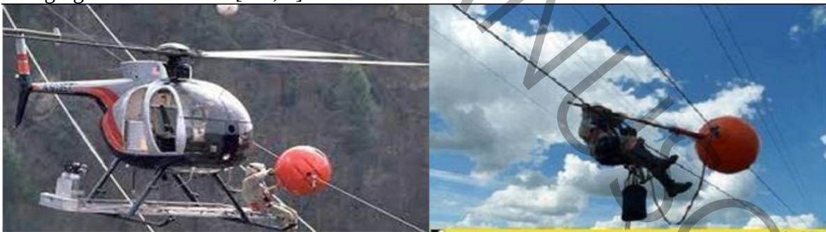
Fig.1. A view of the common methods of installation and replacement of warning spheres
